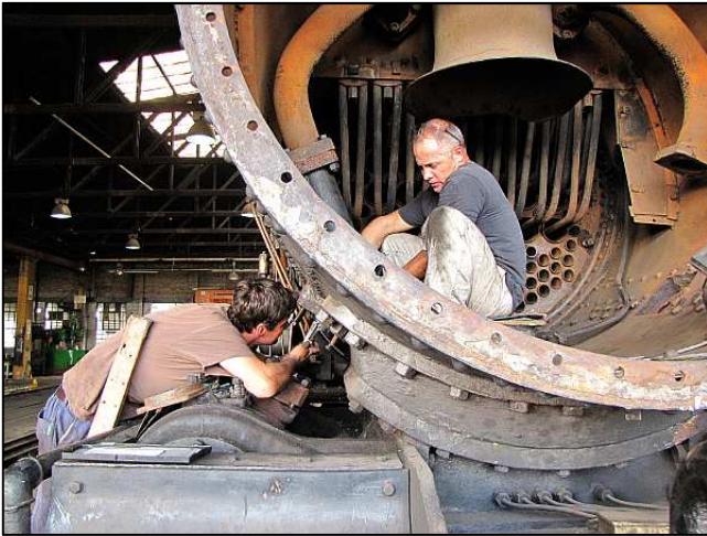
P109 - Locomotive work requires team work, even when the role players cannot actually see each other. They are lining up a tacked-together steam pipe for final measurements before welding – a job made challenging as the pipe bends in two planes.
