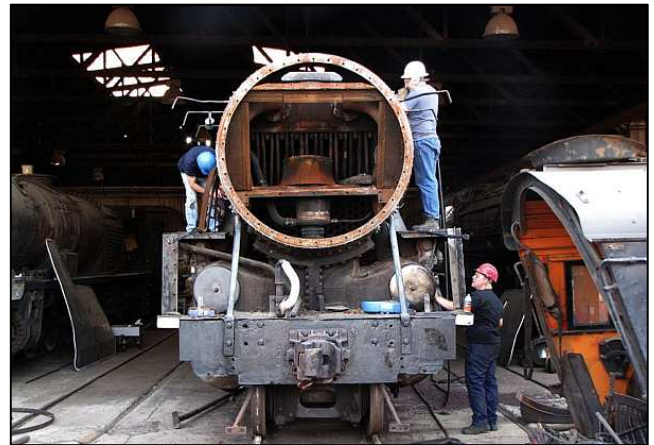
P100 - Because of their size, SAR steam locomotives allow for double-deck work on multiple levels. This locomotive is simultaneously getting etching primer paint applied, old paint removed and baked-on heat resistant graphite paint being removed from the smokebox.
