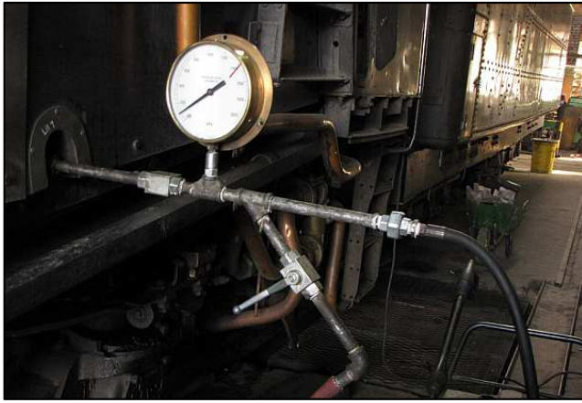
P121 - One of the heart breakers of South African Steam preservation is the mandatory three year boiler ticket, without which a locomotive cannot be fired up. Here you can see a test injection gauge connected to a class 15F's boiler. The cold boiler is pumped up with water and pressurized to 125% working pressure to check for leaks.
