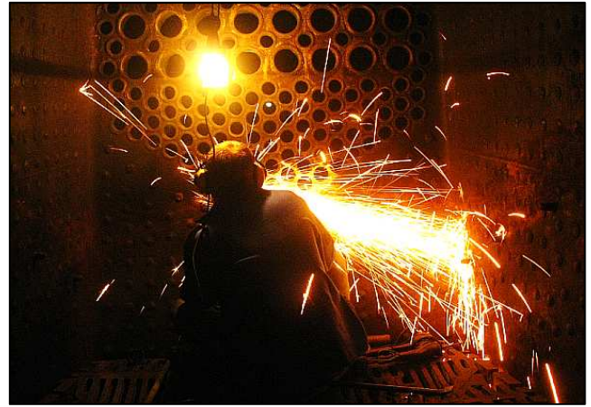
P098 - We often have to work within the dark ferrous sarcophagus of a locomotive's firebox too. This old-fashioned narrow firebox is having the tube plate ground clean and old copper ferrules being removed prior to installing new boiler tubes.
