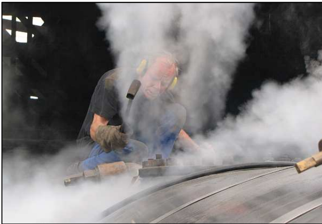
P099 - Some of the work has to be done with the locomotive hot! Here, the safety valves are being calibrated on a newly commissioned boiler. A locomotive's safety valves have to have their settings certified by a Boiler Inspector and then sealed to prevent tampering.
