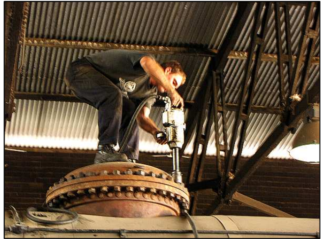
P110 - It helps to not have a fear of heights when in the 15M shops! Perched up on high, Jeandre is going around the 12AR's exposed steam dome with a pneumatic socket driver after the dome's copper sealing ring was found to be weeping during a hydrostatic boiler test.
