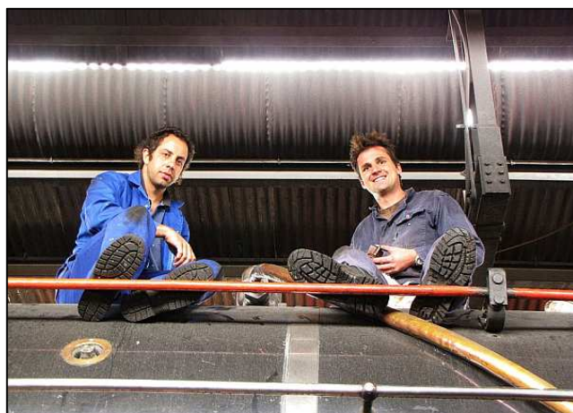
P142 - And you also get them way up on top as well! Andreas (Left) and Dawie are busy inspecting and lapping in one of the boiler's clack valves which has been leaking. They are actually resting their big feet on the regulator rods.
