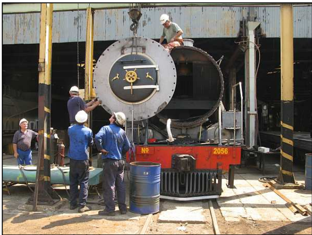
P111 - Here is the traversing crane in use to take the front plate off the 15CA locomotive to start the process of investigating a failed flue. Although the hoist is operated by a pneumatic motor, it is traversed by manual chain drive.
