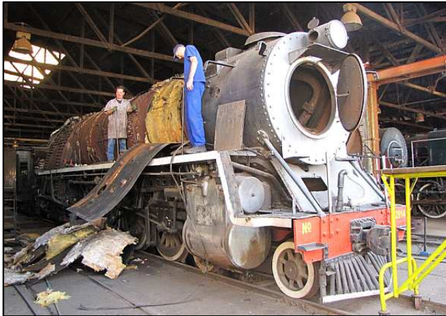
P097 - An example of scruffy and labour-intensive stripping work. Here, the boiler cladding sheets and the underlying thermal insulative lagging are being removed from the boiler shell of Class 15F No.2914 and what a messy, itchy job that turned out to be!
