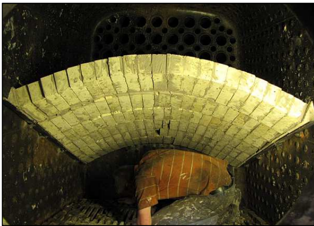
P123 - There is masonry work on a steam locomotive too! This is a brand new fire arch within the firebox of the Class 12AR locomotive. The arch is built from specially angled refractory bricks and cemented together with a special heat resistant mortar. Baked by the locomotive's fire, the bricks and mortar eventually fuse into one solid mass.
