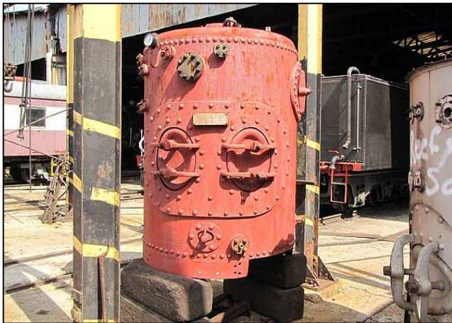
P093 - This is the Cowan Sheldon steam crane's vertical boiler which is in the process of having the leaking rivets of the foundation ring replaced before it can be pressurized with water to test for leaks.
