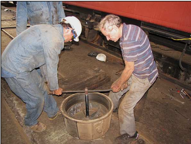
P105 - Although we do have a dedicated coach repair track, it tends to be used for lighter-duty interior fittings, electrical and cosmetics work. Mechanical coach work, such as the repair of the vacuum brake cylinders shown here, are performed in the 15M shop for access to tools and equipment.
