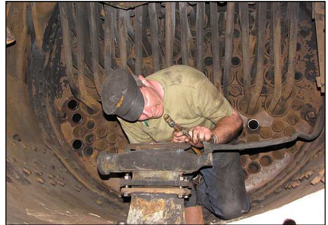
P104 - Not all the work is heavy duty. This fellow is gently cleaning gasket residue off the blower pipe flange and is taking care not to damage the mating surfaces.
