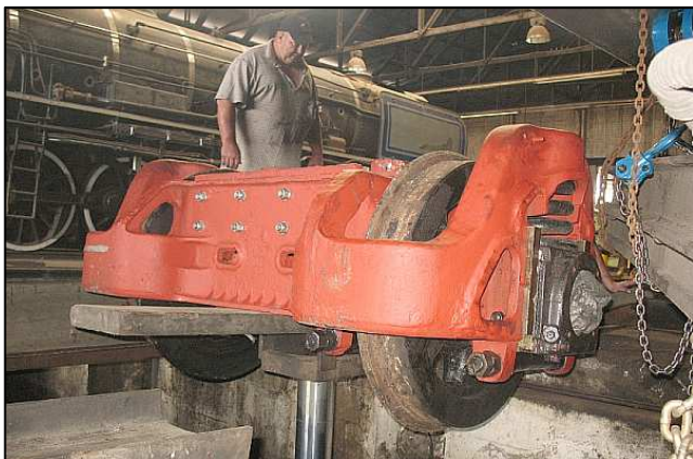
P061 - When we took over the Garratt, both Bissell trucks were unable to swivel for curved track, and the wheel flanges had thus been ground to knife points. The Bissell frames were rebuilt with Vesconite sheeting, based on our successful experience with Vesconite bearings – making this the first time this had ever been done on a Garratt.
