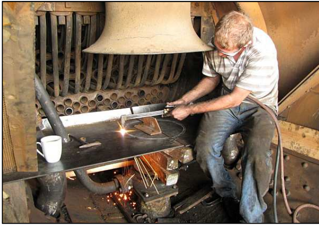
P079 - Some of the cutting torch work is surprisingly delicate. Here, a neat hole is being cut into two sheets of corrosion resistant steel. This would eventually become the 'table plate' which directs the flow of hot gasses. The project was to rebuild the smokebox gear for the Class 12AR locomotive during her last boiler certification in 2013.
