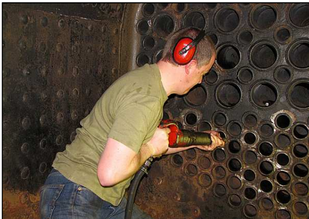
P081 - Along with the air compressor is a range of air wrenches, powered wire brushes, several pneumatic jacks and pneumatic guns. This one is being used to wrap over the ends of new boiler tubes in the Class 12AR's firebox, a process colloquially known as 'beading.'
