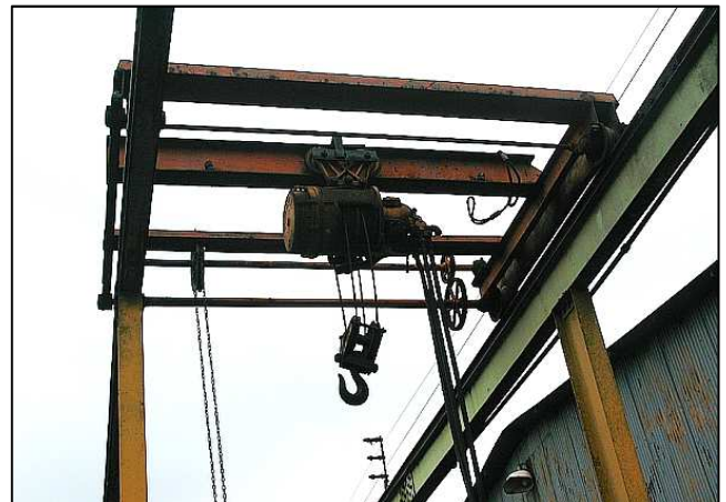
P082 - Also running on our air supply, the manually-traversed gantry crane has also survived into preservation. It serves all eight tracks of the 15M shops and extends into the wheel lathe house. Its main purpose was to hoist and traverse locomotive axles to the wheel lathe for machining.
