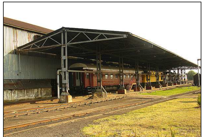
P036 - The boiler washout area was stripped and the steam plant removed, but several tracks, the dual-track canopy and the shell of the boiler heavy-repair shops survived. One of our long term goals is to convert this area into a working station platform for departures and a working steam museum.
