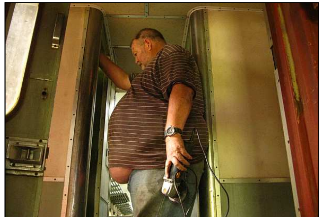
P22 - 'Big Robbie' figures out how he is going to get into that little cubicle to wrinkle the SAR-style 'thunder pot' out. We are going to demolish the left toilet compartment to use that area as a corridor, and extend the right compartment to the middle. Otherwise, fitting a domestic type toilet results in very cramped seating and the door getting in the way.
