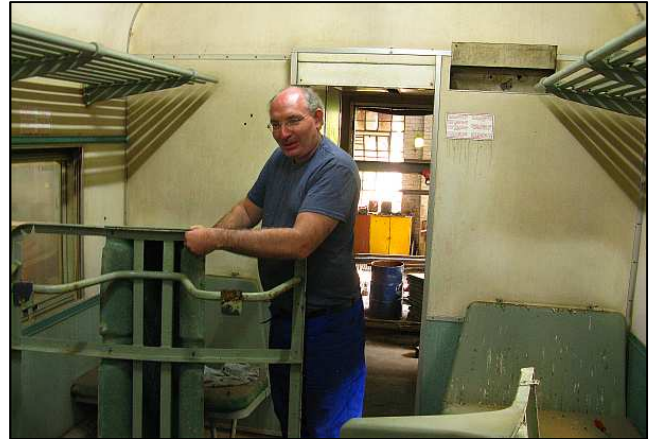
P20 - Aidan brokers a divorce between another seat back and frame. These were each held on with eight bolts and none of them were captive fittings. As the coach was stored with the windows closed, the bolts weren't too bad.
