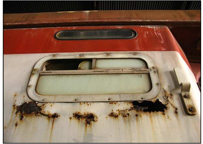
P14 - Here is some bad rust that broke out around a toilet window. This is an unusual location for the rust especially as the toilets don't have steam heaters and it is likely there is a roof or window frame leak letting water into the framing.
