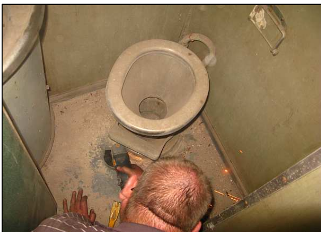
P23 - Robbie patiently grinds away the rusty, urine-corroded bolts holding the flap-bottomed toilet pan down. These little compartments look dingy even when those old laminates are cleaned, and fresh paint doesn't help much. The walls need removal before the new flooring is laid.
