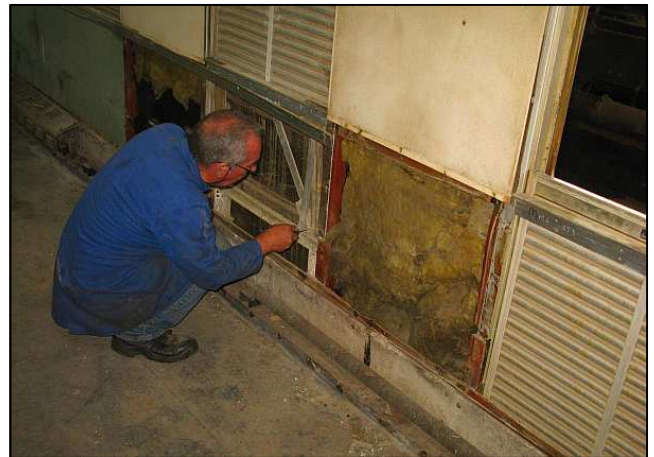
P16 - Gordon wrestles with the jammed counterpoise linkage of a seized window. One of the other windows was smashed. As the louvered shutters are incompatible with the sleeper coaches, they will now remain where they are!
