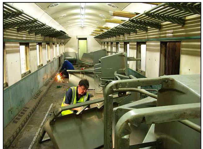
P18 - This was the second coach interior stripping session. Nicholas is seen gamely working away at the BIG jumbled pile of 3 rd class seats – all of which were cleared by day's end. In the background, Gordon is grinding away the corroded bolts that retain the steam heater skirting covers.
