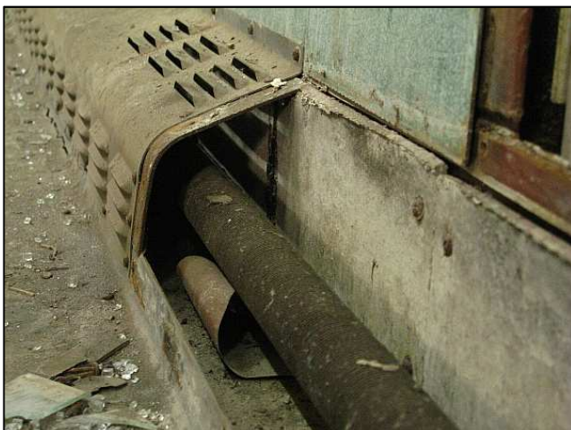
P17 - To get the wall panels off, the steam heater covers had to be removed, leaving this 'cross-sectional' view of the densely-finned heating pipes. These have caused rust in many coaches through rising steam from leaks and we are removing this obsolete equipment on any coach we rebuild.
