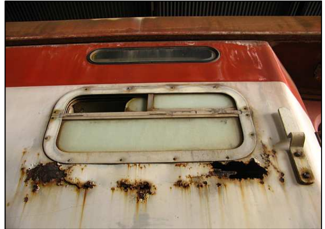
P14 - Here is some bad rust that broke out around a toilet window. This is an unusual location for the rust especially as the toilets don't have steam heaters and it is likely there is a roof or window frame leak letting water into the framing.
