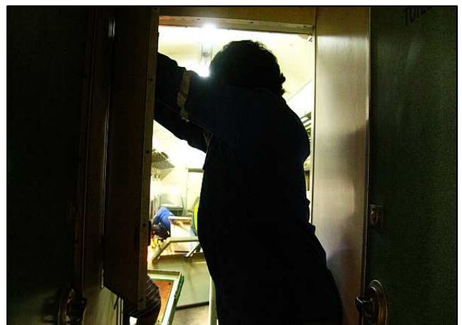
P24 - Alan's FAVOURITE position – elbow-deep inside a live distribution board. The vestibule lights will need to use converted existing-style fittings as the high-efficiency integrated fitting used in the interior are now only available in 2ft lengths, too long to fit into the existing recesses.
