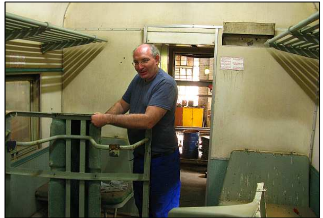
P20 - Aidan brokers a divorce between another seat back and frame. These were each held on with eight bolts and none of them were captive fittings. As the coach was stored with the windows closed, the bolts weren't too bad.
