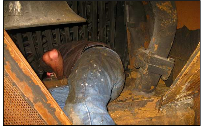
P02 - Smudge in da box. Shaun checks apprentice steam fitter Jeandre Gordon's boiler washout work before authorizing the baffle plates and spark arrestor grids to be refitted. (Which would obstruct access to the tube plate.) He is checking the front tube plate washout plugs here.
