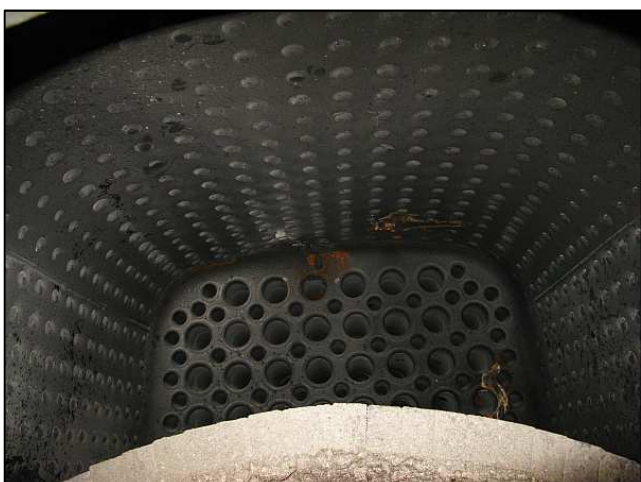
P05 - A quick peek into the firebox shows that the relatively new fire arch isn't in bad shape. But there is a weep from the right front fusible plug and from one of the boiler flues as well.
