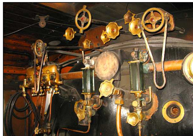
P04 - On the boiler backhead within the dark cab, there is just a blank circular wooden patress where the boiler pressure gauge would be. Although not necessarily a task within a standard boiler washout, the gauge was removed for repairs and recalibration. You can see the rear corner of the crown sheet through the washout plug aperture.
