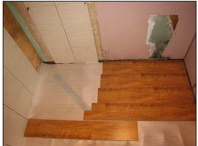
C14 – While the silicone cures behind the tiles, the foam under-floor sheet (with integral water proofing membrane) has been laid and Alan Lawton had started putting the new laminated T&G flooring in. The toilet's waste pipe will be re-routed through the wall to eliminate an extra S-bend.
