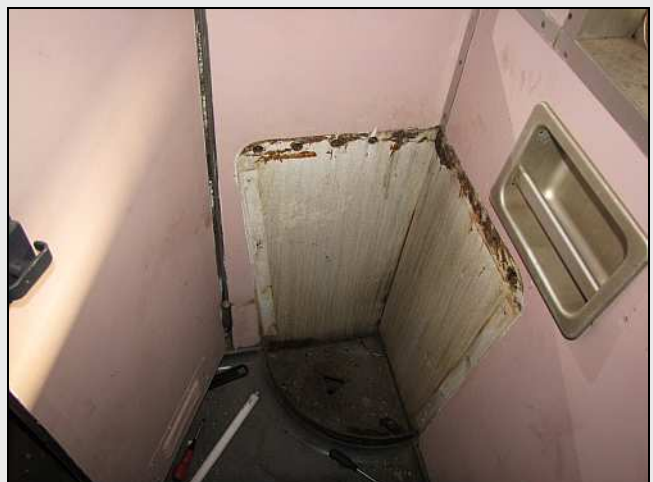
C28 – Generously-built Robbie Davis-Hannibal had to fold himself into this small space and strip the original bathroom. Once cleaned up, this room will become the lockable linen store for when the sleeper train is out of use.
