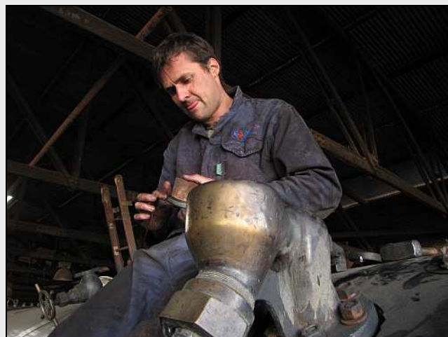
F04 – Dawie is applying grinding paste to the vane element of the clack valve in the foreground. We normally grind 'em in lightly and then apply silicone to the valve seats to prevent false boiler leak readings. But Dawie had spotted a flaw in the valve seat and trying to cut it down.
