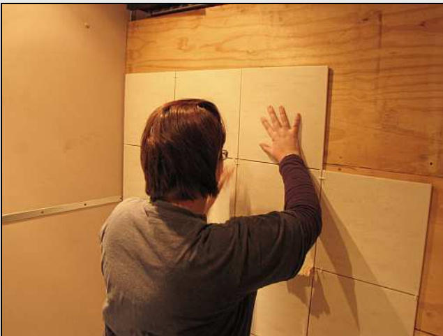
C09 – Lauren 'Smidge' Ackerman is placing the splash-back tiles in the center bathroom. They are being fastened with generous blobs of clear silicone and will be grouted with white silicone. The silicone will impart some flexibility to the hard ceramic tiles on a moving, vibrating coach.
