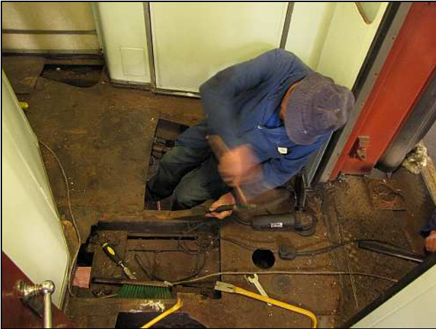
C07 – The consensus is that we will lay the new plywood sheeting directly over the access holes, but with a coating of bitumen on the undersides and along the edges. To minimize unsettling floor flexion under heavy people, we'll span the holes with a piece of scrap angle iron welded in.
