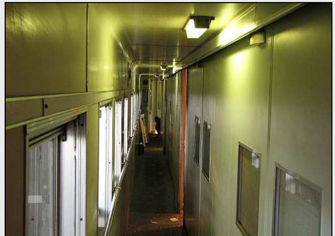
M04 – A view down the Gold Class corridor at Gordon grinding off endless welds. The entire floor has been stripped and now it acts like a big fly-trap. If you don't keep moving, your boots literally stick to the glue left on the floor!
