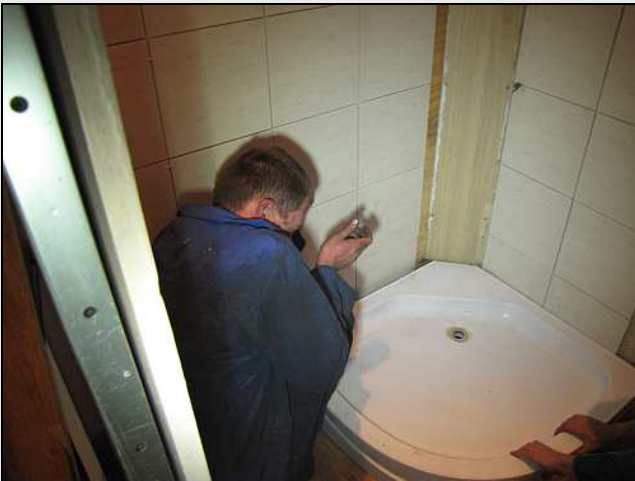
C21 – Because this bathroom floor was now physically higher because of the extra layer of 7-ply plywood sheeting that had been fitted, and then the laminated planks, that corner panel had to be trimmed to fit the pan. It was still a bit long, so it was trimmed twice more.
