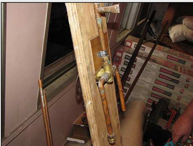
C17 – A little extra work involving saddle clamps and some scrap flooring as spacers makes for a more rigid mounting. At least one of these showers had already started to leak due to fractured pipes. Note the stray tee-piece .. not ours!
