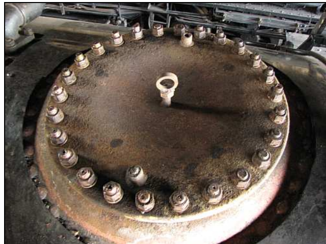
F02 – The 'dome cover' on the 15F's is actually a manhole manhole cover. Noticed the concave dishing to withstand the pressure. Those nuts all need to be tightened with an air gun before the boiler can be fully pressure tested.
