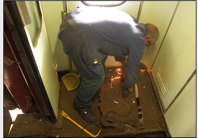
C02 – As Gordon worries away at a nearly-cut plate, you can clearly see the corroded edges. The water was getting into the floor timbers from underneath, as well as through the bathroom, open doors and the gangway drips.
