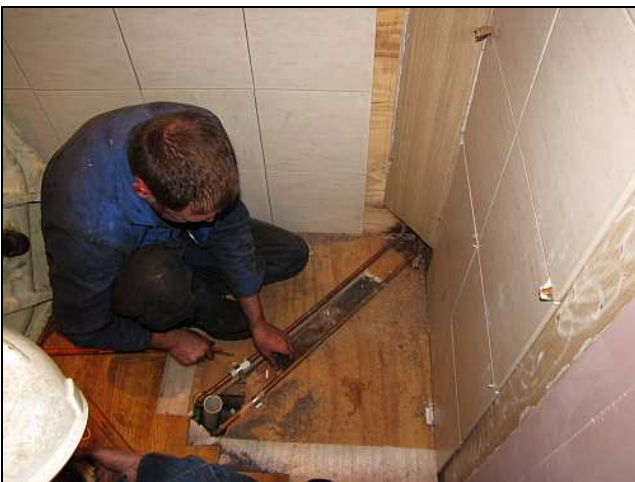
C23 – A part of the customization that will need to be done for each shower. Dr. Smudge uses a crow bar to peel off the floor vinyl remaining in the drain trench to provide clearance for the PVC drain pipe. Note the lack of a drum trap or U-bend – not necessary for external discharge.
