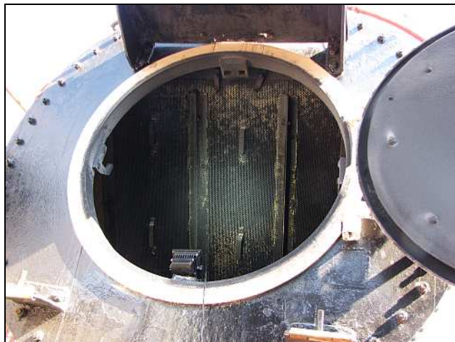
W02 – As the front tube plate is known to be wasted, the 12AR Loco is on a strict cleaning schedule to forestall any further sulphur-leached corrosion from wet char and ash. The smokebox gets cleaned after Every ... Single ... Trip.
