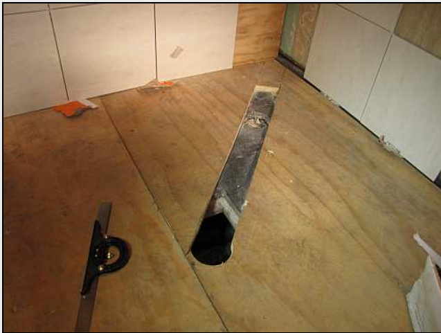
C13 – The shower drains are to be rigid PVC pipes rather than flexible stuff – this trench will also house the water pipes. Each coach's shower drains will need to be reconnoitred in advance, due to framing and bogies getting in the way. They also need to fit beneath the shower pan.
