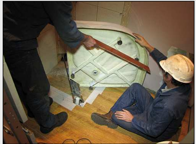
C20 – Fitting the shower pans proved to be tricky with SIX adjustable feet to set up level, and with the pan tilted by the planking too. Note that shower water pipes had already been brazed in – joints above rather than below floor level.
