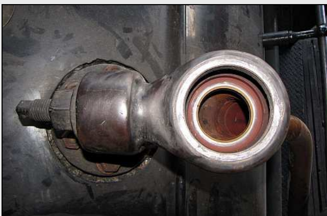
F05 – Looking down into the clack housing, you can see the flaw at 10 o' Clock on the valve seat. (The dark spot.) The clacks are self-cleaning, as they spin when they lift. But that's to deal with water-bourne scale and impurities and isn't capable of resolving damage to the valve's seat.
