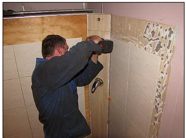
C18 – Smudge Ackerman fastens the corner panel with the same self-drilling screws used for the skirting boards. The RHS bolts had to be angled perpendicular as that firewall has two sets of laminated ply astride a sheet steel plate.
