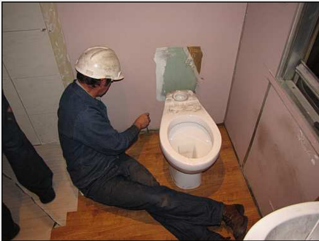
C25 – We will be re-using the close coupled toilet pans that were originally installed by Setimela, but with better quality seats. The fellows were debating putting the toilet in the center line for more leg room on the user's left side, but the route for the waste pipe dictated the offset position.
