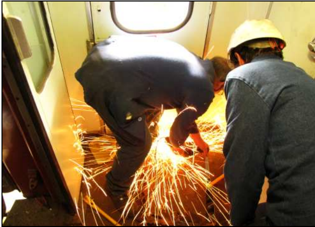
C01 – Inspection of the vestibule floor under-plating through the cut-outs in the timbers made by Simon revealed that the plating had corroded under the ply-wood sheets. Today, all of the timber and plating was removed.
