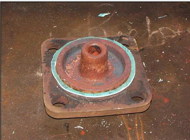
F09 – All alone and neglected in his dimly-lit, oil-scented cave, Aidan McCarthy made up five new Klingerite™ gasket rings for the regulator spool covers – 4 mains and a smaller one for the pilot.
