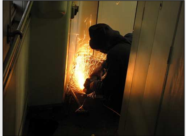
C08 – With that decision made, work continued on chiselling away the leftovers from the hole covers and grinding down the welds. In spite of the planned bitumen, the floor boards will also be mechanically held down with cadmium-plated countersunk screws.
