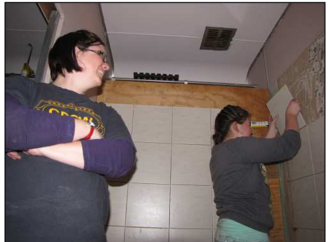
C10 – This awkward shot, taken from ground level through the window, serves to show a better rendering of the neutral tile colours chosen. At work is Cheylin Blore, Lauren's eldest of three. The bare space in the corner is reserved for the pipe risers and mixer valve panel.
