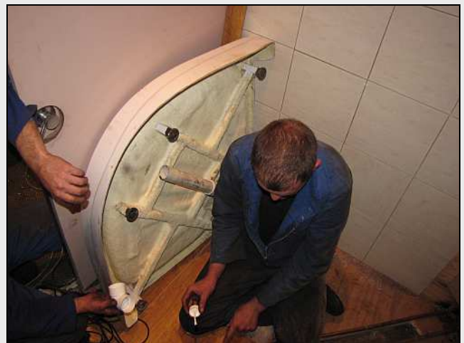
C24 – The drain pipes were put together with proper liquid adhesive for PVC for a true chemical bond, rather than just any old glue ... or even silicone! It made for some mad dashing though, to try and fit the vertical pipe up from underneath before the fusing PVC had time to set.
