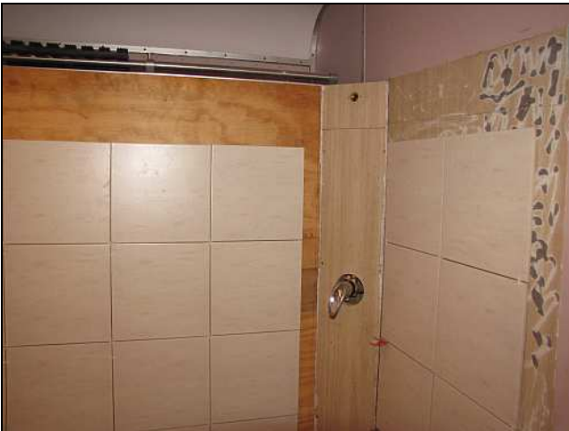
C19 – The outlet pipe for the shower rose is threaded, not soldered, so the shower heads can be removed later on. We are going to try out a low pressure high flow 'sunflower' type shower rose on the pumps before purchasing more.
