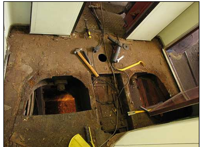
C04 – Here is the vestibule floor with the under-plating removed. The steel visible here is a part of the coach frame. It needs to be de-rusted, cleaned and primed for a new floor. The big nuts are for the buffer-plate rams.
