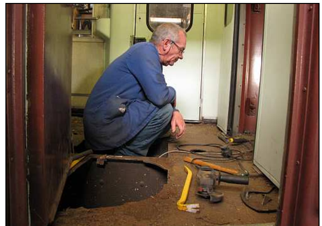
C06 – Sitting on the draft cushion stack, Gordon is thinking things through. If we plate this floor with our stock of thicker plate, and then put new plywood on top, the higher floor will foul the inward opening doors. It is also one of the reason why cheap vinyl was originally laid – it is THIN!
