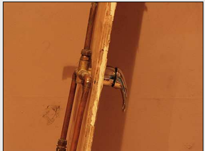
C16 – Classic plumbing by the now-failed Setimela Tours Company. Neither the pipes or the mixer valve were physically attached to the timber. They had relied on two screws through the plastic escutcheon plate for the mixer, and on the shower rose's pipe to hold everything together.
