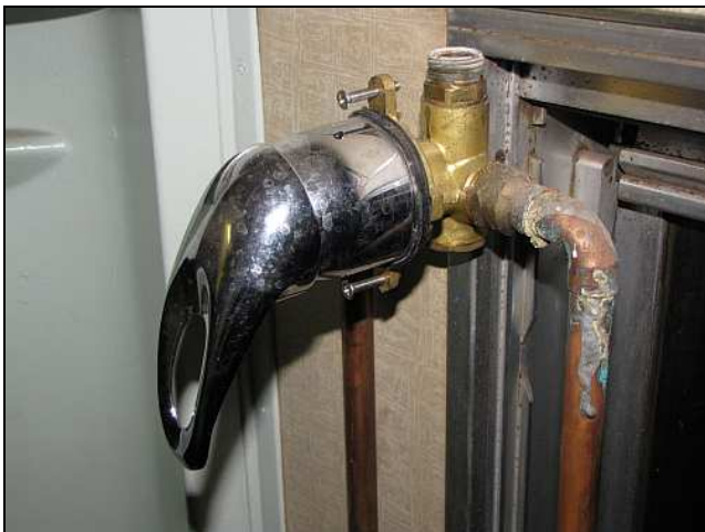
C15 – Leaning loose in the corridor, this is one of the modern shower mixer units that had been purchased and installed by Setimela. They aren't bad quality and have seen little use, so we are going to reuse them. We already know they fit in the corner panels.
