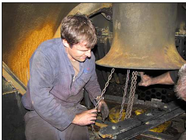
P08 – Dawie has a first attempt at untangling the loose-hanging looped chains of the hoist before looping them around the clench bars.
