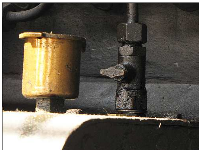
P16 – Close-up of an oil cellar and one of the steam cylinder oil line choke valves on the Class 12AR. The latter could have done with a good cleaning!
