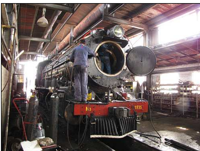
P05 – The 12AR gang are discussing removing the petticoat for better access to the holed superheater. Dawie is moving a shaker lever to hang a chain hoist within the chimney to support the loose petticoat.
