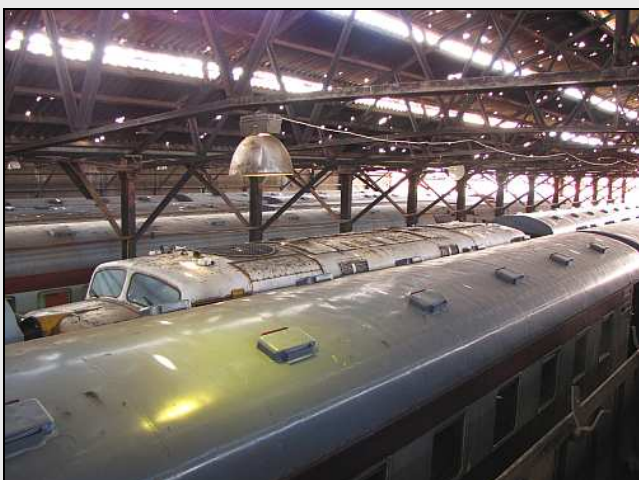
P23 – Sandstone's DE2 Diesel waits amongst the coaches. It isn't coping well with the hail-damaged roof letting in the rain. We will cover the diesel with the wheel lathe's tarp before the next rainy season.
