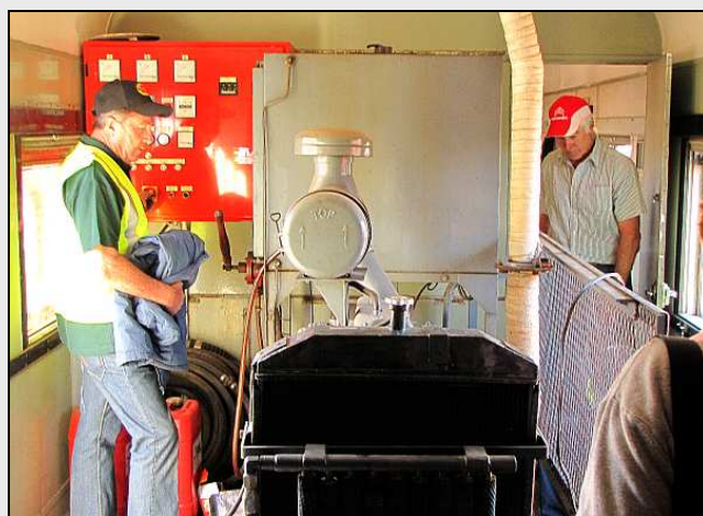
P112 – A bit of consternation going on here as the generator would not start. It turned out to be bad starting technique, as you need to lean on that starter in a long burst to build up enough compressive-heat to get the diesel fuel ignited. This diesel engine doesn’t have glow plugs.
