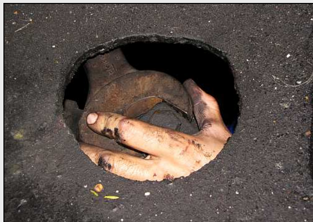
R04 – Ooh and there were some naughty Afrikaans words coming out from under the running board when the time came to open and service the non-return valves. The standardized valves are too tall for the piping center line.
