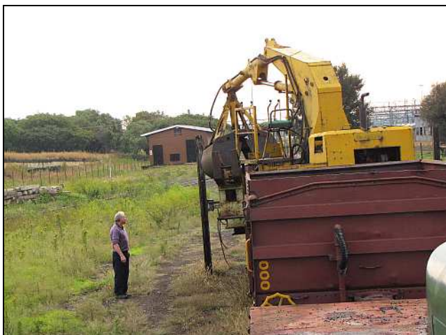
S09 – Nah, it ain’t gonna make it. The grab bucket got through with bit of a scrape but the control panels didn’t. I thought we’d end up torching the panels off but instead we wrestled that pole and had it laid down flat to the ground.
