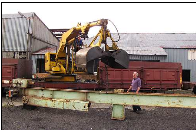
S05 – On 13 th April, we had to 'swagger' the lower half of the swager in towards the rails. It was delivered by road truck, hence the awkward angle. Care had to be taken not to roll this lot over, as it is top-heavy on those pedestals and the foot flanges tended to dig into the soft ground.
