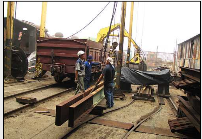
S04 – In this view, the double C-Beam construction of this large but simple machine is obvious. The use of wood blocks eases the slinging in future. The second half would have to be unloaded without the crane, as these guys had unavoidably taken that unloading spot under the gantry.
