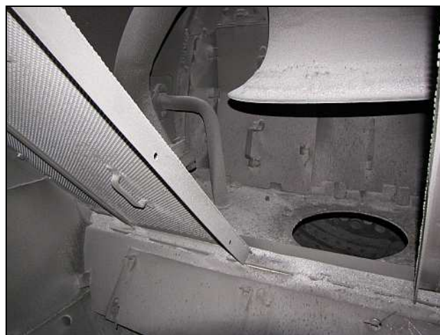
B08 – Showing the cone's aperture in the brand new table plate. The flue gasses are deflected downwards via those solid baffle plates, passing under the table plate and around the angled lip. The centrifugal force at the change-of-direction throws out the char against the smokebox front plate. The final exhaust gasses actually flow from front to rear through a bank of perforated spark arrestor grids.
