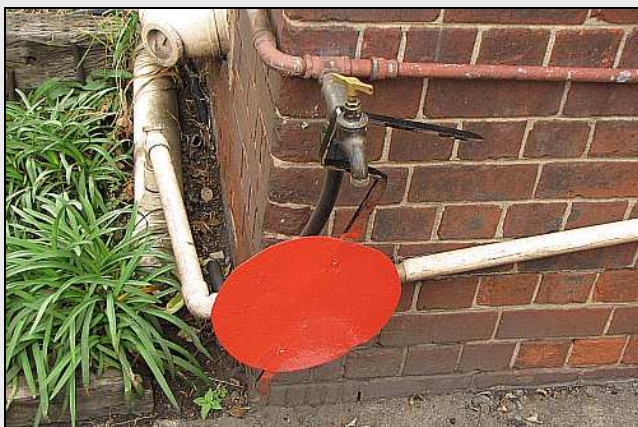
M03 – NOTICE : This Water Tap Is Presently Under Repair And Must NOT Be Moved. By Order : Attie De Necker.
