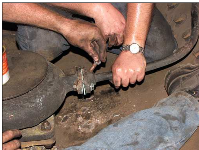
B05 – The blower fault turned out to be a loose flange and a matching blown gasket on the outer end of the blower’s steam pipe. In amongst the many assorted tight-schedule jobs and the late night on 9 th March, the bolted flange on the other end wasn’t tightened properly. Oops!
