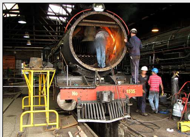
R16 – More pyrotechnics on the job as Dr. Smudge cuts away the rusted-on nuts from the waist flange. The new nuts will be 'copper-slipped.' (The 'oud Spoories' used graphite in a vain attempt to stop threads from rusting.) The table plate and baffles are to be rebuilt from abrasion resistant-steel sheeting and the bolts treated the same way.
