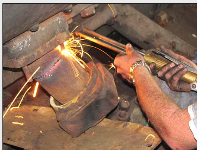
R12 – The cutting job was going well – a bit TOO well. It turns out the whole steam pipe has thin walls and it was sagging under its own weight during the cut. Note that the plastic tray protecting the valve chest inlet had been replaced with something with a MUCH higher melting point!
