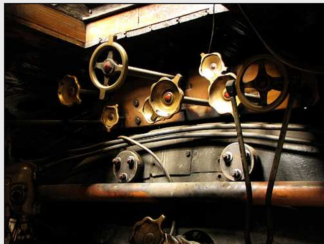
M04 – Second-hand light on the spindle board of the 12AR No.1535 parked under a translucent roof panel. The water columns have been removed and blanked for hydraulic testing, although the pressure gauge has since been fitted.
