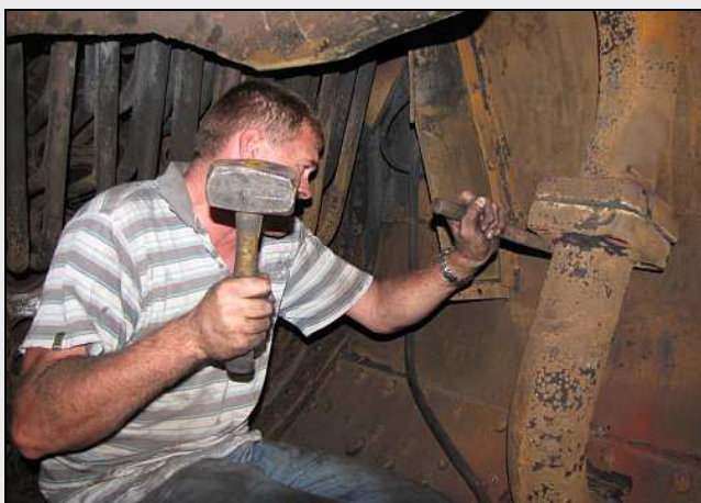
R17 – You need a really delicate touch to work on an SAR steam locomotive. This job required acetylene, a welder, 6ft cheater pipes, big mallets, slogging spanners, a sense of humour and several cups of tea – all in a day's work!
