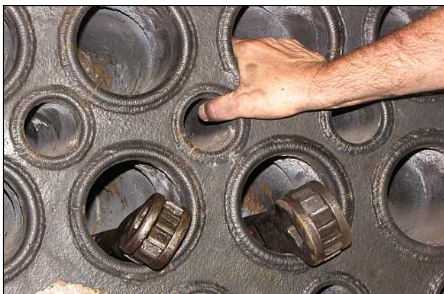
B05 – A nice clean rear tubeplate shows the end results, how the tubes and flues are beaded over and then welded. Superheater flues make handy built-in tool storage pockets.
