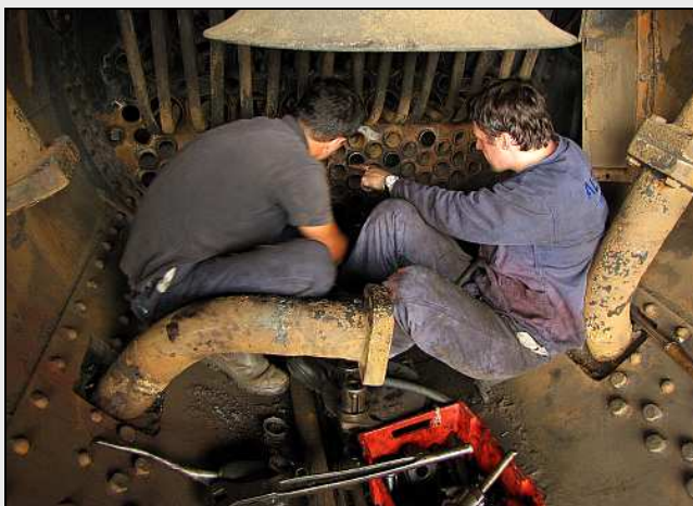
B11 – Sitting room only. Although there is more light and air available at this end, it is also a bit more cramped. Dawie and Michael discuss what to do next. All the boiler tubes need to be installed and expanded-up by the weekend 26/27 th Jan. for a preliminary Boiler Hydraulic test.
