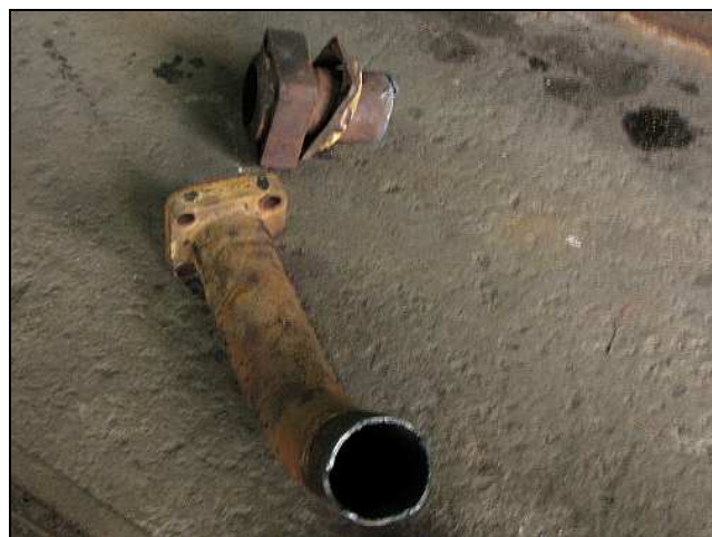
R14 – The RHS steam pipe is definitely thinner than the left side. So either some long-ago fitter took a short cut or the pipe has been replaced before. We aren't even going to bother to check the pipe – just getting sections made up and bent for decent quality replacements. (On both sides.)
