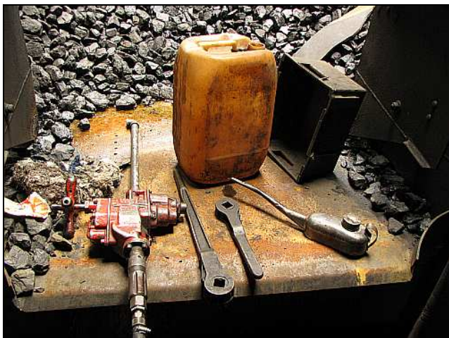
M03 – Some tube expanding stuff laid out on the 12AR's now-rusted shovel plate (leaky roof panel) and I could hear echoey grumping from Dawie inside the firebox. It turned out that I was standing on his boxed vernier calliper. Oops!
