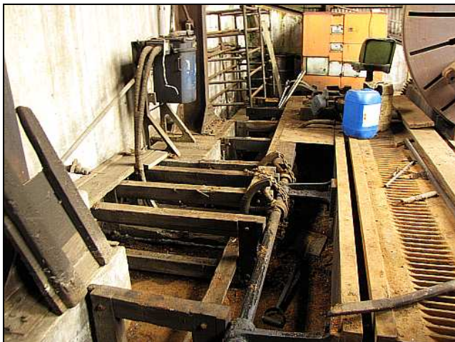
W07 – The old floorboards were lifted and decades of debris and lost tools were shovelled out once the ‘sump water’ drained away. (The spade is not exactly OEM!) In the center is the ratchet-operated tool feed shaft which connect via chains set into those quadranted sheaths.
