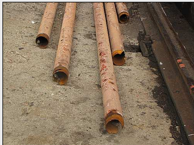
B02 – A view of some of the old tubes that were pulled out. You can see how the tube ends were chiselled to split and collapse them – they are ‘only’ restrained at the front end by friction via expansion. Once the rolled-over ends at the back-end (the beading) and its welds are ground away on the tube plate, the old tube is free to be withdrawn.
