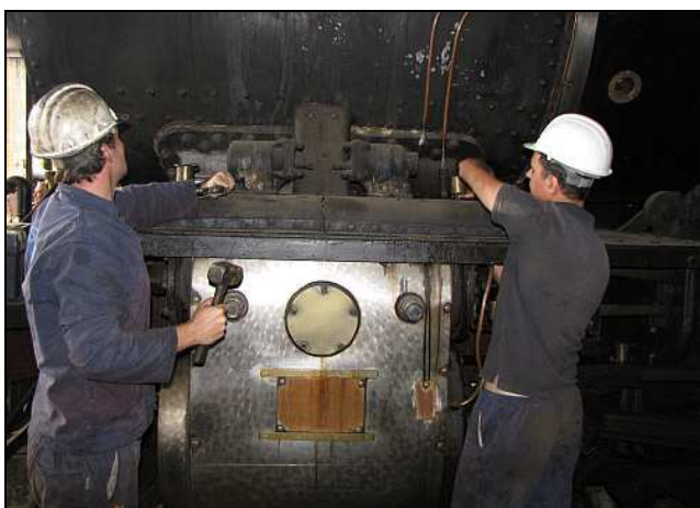
R15 – Dawie (LHS) and Michael, both being taller than Johann Breydenbach, are able to strip the left cylinder area from ground level. It was decided to remove the still-intact LHS steam down-pipe anyway while we had still access and we may as well have two new un-worn pipes made up to the pattern. (Mirror images of each other, of course!)
