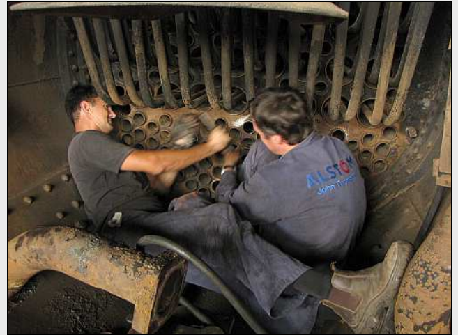
B14 – Double-beat ratchet action. Because of the lack of room within the smokebox barrel, it was easier for each fellow to brace-up in his own direction and pull the ratchet his way. That resulted in this very cosy-looking scene.
