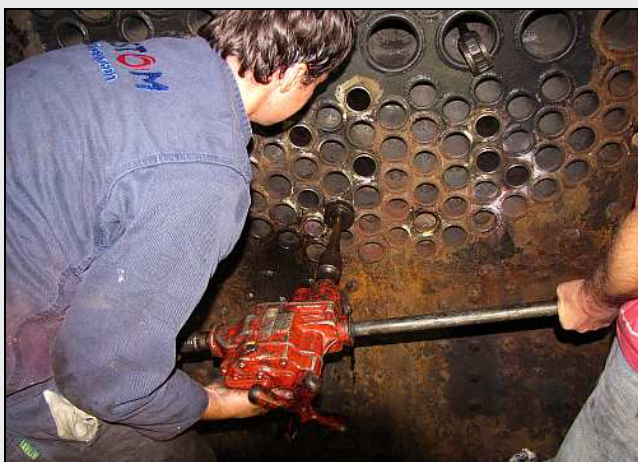
B07 – Once the mandrel and the expander are matched up, the air-motor can be attached. The job usually has to be done in several stages as the expanders are exchanged in stages for bigger ones as the tube-end expands into the aperture. Doing the job too fast will tend to split the tube.
