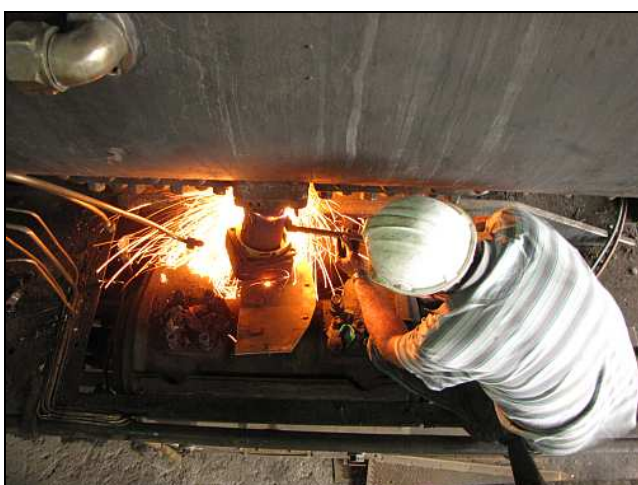
R11 – A top view of the pipe cutting in progress. Of interest is the bundle of small bore-pipes at the left. Two of them are condensate drains for the reverser’s power cylinder, one is a condensate drain for the vacuum ejector exhaust line and one is the discharge for the reverser’s valve chest.
