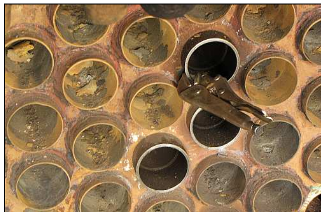
B04 – Boiler tubes are not only damaged by corrosion, leading to perforation, but are also worn by char cutting. You can clearly see how the old tube ends are worn down compared to the new tubes. The 3 new tubes had already been expanded into place and you can see the inner ridges which mark the inner face of the front tube plate.
