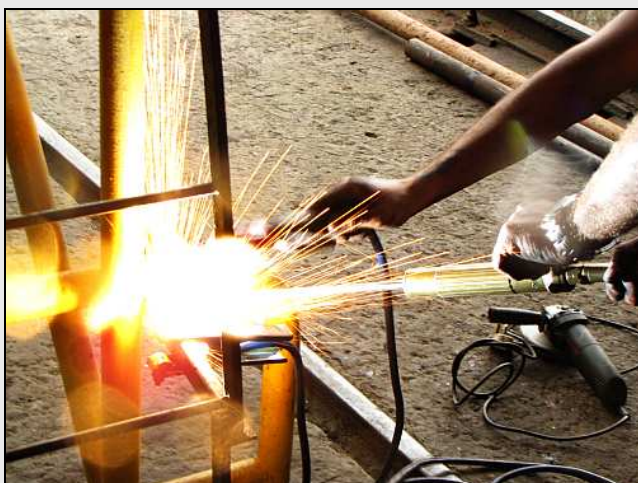
R09 – As I rarely ask the guys to pose, and I take photos under less-than-optimal conditions, I discard about half the photos I take. But occasionally I do get it right, like this moment that the cutting torch is ignited with an arc welder.
