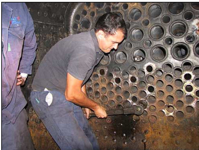
B09 – Michael does the final crunch-up using the ratchet driver on the square shank. In the final stages, hand tightening gives you more control. Also, using the air-motor can be dangerous at this stage, as it tends to kick back while running at full power driving the now-tightened tool.
