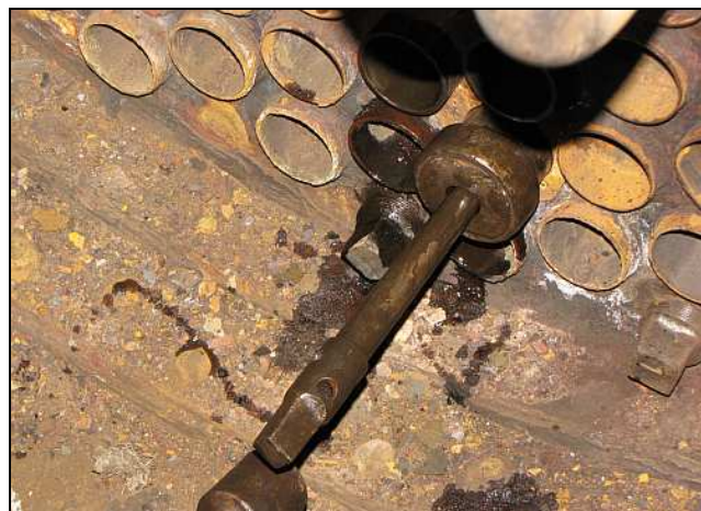
B12 – This tube would give hassles as the end is protruding a bit too far and is blocking full penetration of the expander. They could have cheated by putting in bigger mandrels but that would have belled the end out. Instead, the expanders were changed more frequently than usual.
