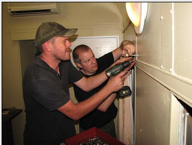
P27 – Look at those grim faces! Fitting new curtains proved challenging as the previous rails were mounted over stainless steel plates which baulked the self-drilling screws. We had no decent drill bits of the correct size either.
