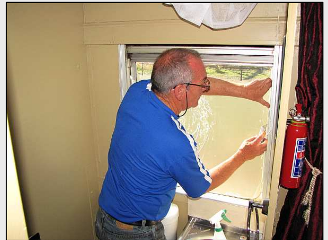
P22 – Gordon applies the opaque window film to the bathrooms. He struggled at this time of day, as the warm afternoon sun was prematurely drying out the slippery detergent upon which the plastic film would slide.
