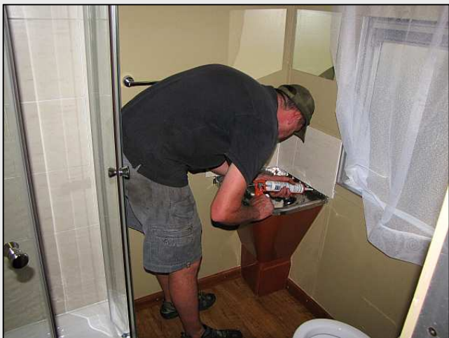
P23 – Smudge Ackerman completes some last minute sealing work on a sink splash back. He was getting a bit stressed at this point as there was still a silver class coach in the 15M shop which was waiting to have the toilets fitted, and the sands of time were running free and loose!
