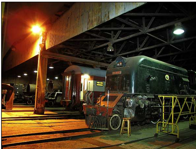
P47 – The bad electrical phase was energized later on, leading rise to this scene in the old 15M workshop. It looks quite busy – but there isn't a single person in sight.
