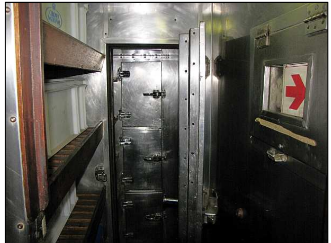
P16 – A view into the walk-in refrigerator, which was being pre-cooled for the tour. Although functional, the cooling plant wasn't quite up to the load and the Feedem people had to be careful about selecting cool storage. An extra deep freezer was loaded onto the S&B van to add capacity.
