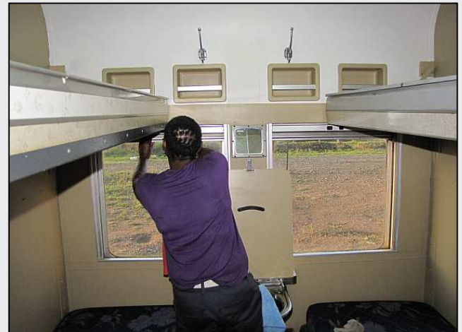
P34 – As some of our staff hadn't been able to keep up with their finishing work during the week, the good ladies of Crystal Cleaners gamely got stuck in with cleaning paint runs and splats from the bright work. Technically, it wasn't their job. Pictured here is an Economy Class Compartment intended to sleep two with the top bunks used as shelves.
