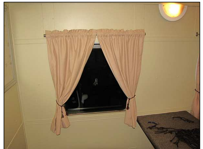
P28 – Mounting the dining coach curtains required scraping the paint and plaster back to find the original holes. We later got a three man 'assembly line' going to fit and decoratively knot the new tie-backs.
