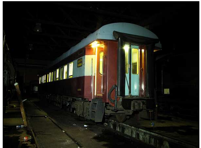
P46 – Coach work in the dark. Shaun Ackerman would continue working alone through the long night to install the toilets and bathroom fittings on this coach. Most of the other guys were sent home to be able to do their packing.
