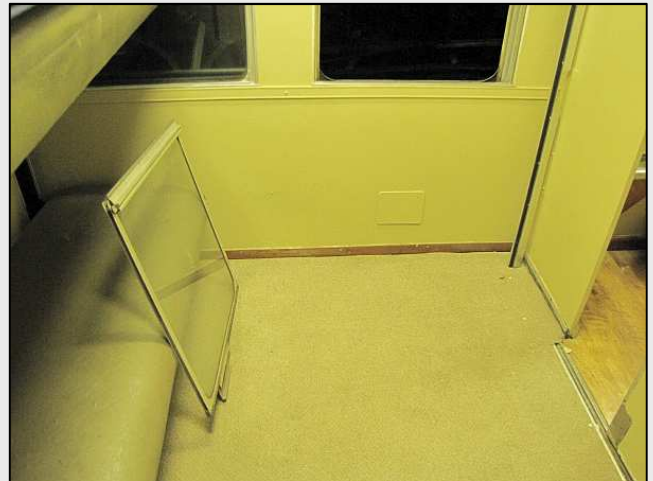
P44 – A silver class compartment with one window pane removed to allow the loading of a chair. The beds still needed to be adjusted outwards and Shaun Ackerman was then-currently installing the porcelain toilets.
