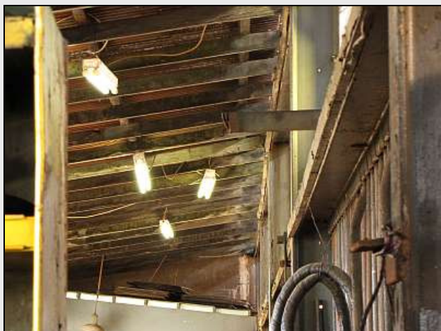
M03 – The 'interesting' wiring at the depot is gradually getting sussed out! These old lights have been restored to action by tapping power from the ex-upper-machine shop DB, and the other (corroded) end safely terminated. How nice it is to have ample lighting in the oil store and not to have to TASTE the difference between Steam Oil and MH!
