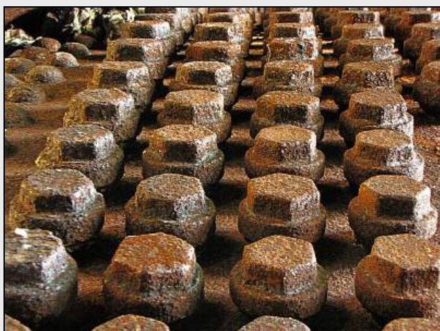
F05 – It is unpleasant work to expose the stay caps – rusty, sharp-edged cladding plates to be removed and obnoxious thermal lagging beneath. Many of the plates were welded together instead of being bolted to the crinoline bars.
