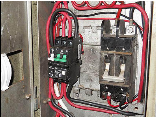
C03 – The ‘Semuma Coach’ is being upgraded to use 220V power, like all the other coaches. The size difference of new distribution board hardware is remarkable – showing several decades of development of MCB switchgear.
