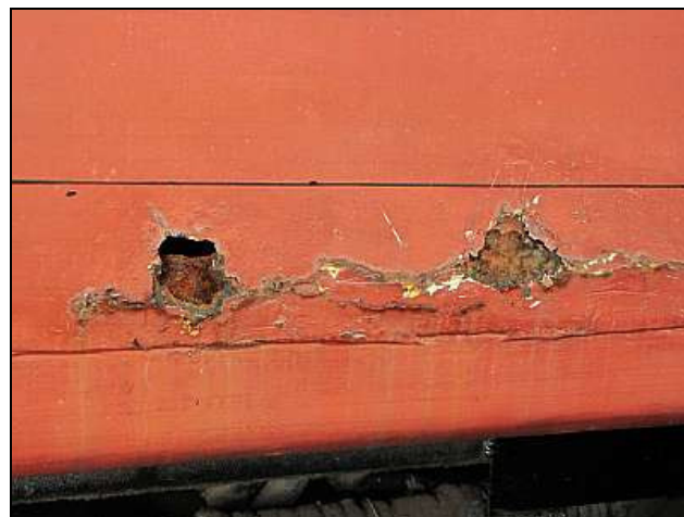
C10 - A lot of our coaches have this sort of damage above their footing rails. It is caused by leaks and condensation from the steam-heat lines within the coach. The bitumen sealing also tends to fail here, providing close, laminated layers that wick up the condensate and rain water.
