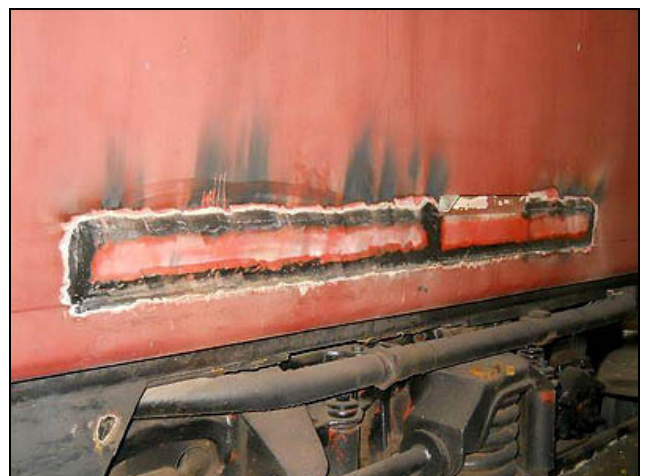
C06 – A newly ground-down MIG-welded patch on the Sandstone Sleeper No 28332. As the base metal is more sound on this coach, it is being used to fine-tune the tricky combination of welding techniques that are required.
