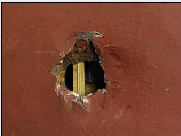
C09 – Tin-worms usually pupate after monsoon season and then fly away, leaving characteristic chewed holes. A common starting point for the rust are the drainage paths from the inset and unsealed window apertures. Seen here through the hole is a window glass runner.
