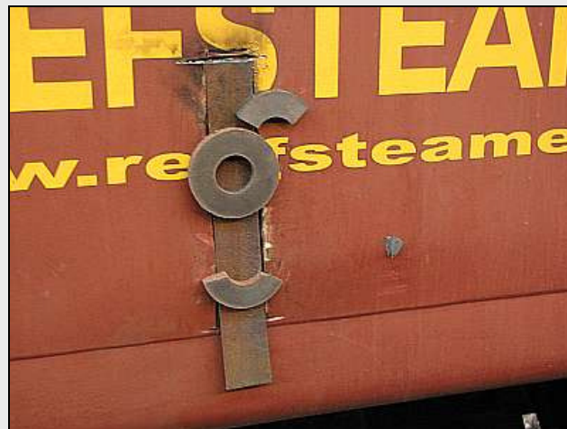
C08 – A assortment of magnets hold this patch in place, so the measured steel doesn't go astray. This scary looking hole started as a fine vertical crack over the frame – and ever-more rusted metal was revealed when it was cut back.
