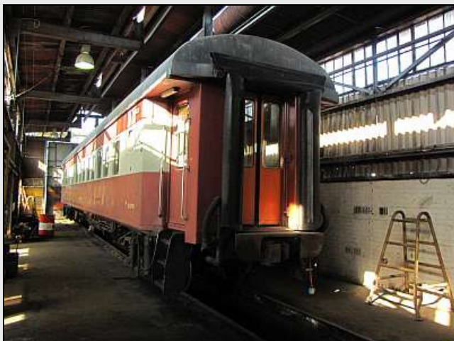
C13 – An unusual sight, a coach in residence in our adopted Running Shed. The Sandstone Sleeper has been parked undercover to keep the wind from interfering with the welding work – which is presumably tricky enough!
