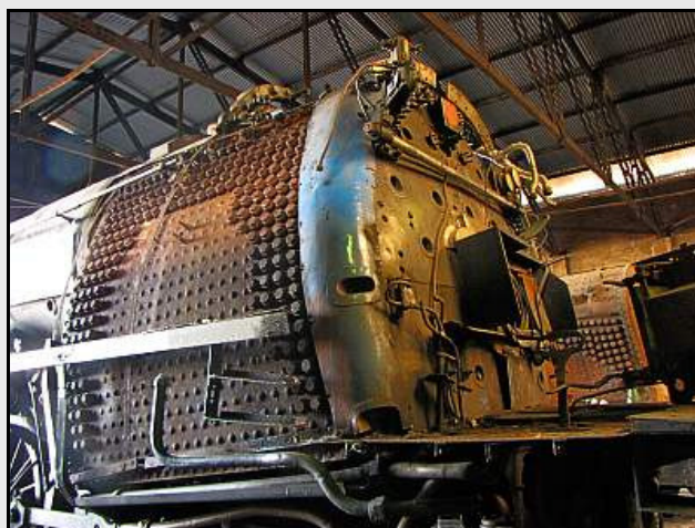
F04 – Aidan McCarthy has been keeping himself busy by removing the cladding from the left flank of the firebox. You can already see some revealed lime scale streaks from stays and stay covers that were once leaking in service.
