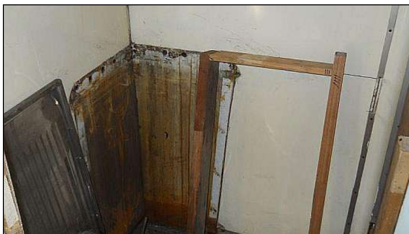
C16 – Here is the still rather raw scullery area being made up for the 'Locomotion' coach. The stained area on the wall is where the corner basin used to be. The coach boys are planning to do some much-needed surface preparation and then to apply white enamel paint to the whole compartment ... before installing the new sink. They might even rip out the old toilet floor pan and put in something more robust and waterproof.
