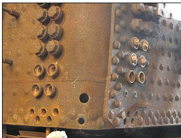
F06 – Some clean-up work still required. Some of the truncated foundation ring rivets need to have their outer ends removed. Two stay cups got bent in the process of whacking out rivets too. Note the cladding's crinoline studs.
