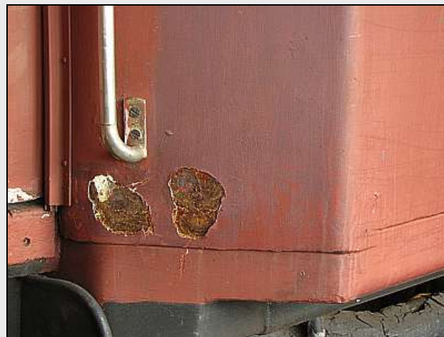
C12 – One of the few examples of external rust on sound plate work. It takes a good workman to resist the temptation to just patch and paint over a rust hole instead of bravely cutting back. But a bodge job just won't last on a steel railway coach, especially when parked in sun light.
