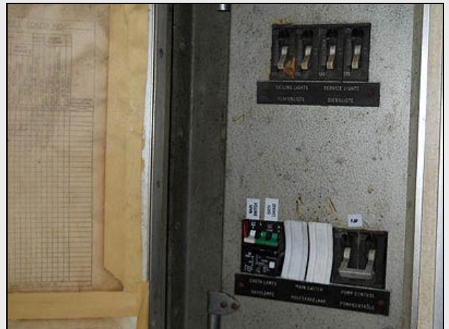
C04 – An external view. As the coach only has a single cabin instead of multiple compartments, the board is relatively simple. Notice that the Earth Leakage is an isolator (green) – the mains is protected on the live side.
