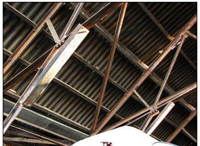
M12 – Unnoticed detail. Loco-blast deflector shields are still protecting the steel beams in the old running shed.
