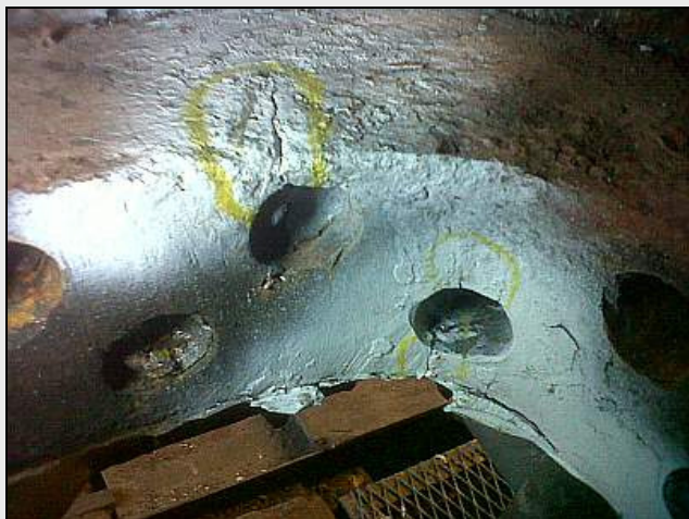
F02 – As revealed by the MPI, here is the crack damage to the foundation ring. We were already aware of the lower crack, which goes right through the rivet hole. And there are fractures in the center of the steel mass above the hole.
