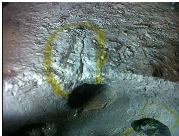
F03 – The other 50mm long crack from the top rivet hole was a surprise to us. Fortunately, it is easy to reach for welding. This crack leads directly into the water space between the inner and outer firebox plates.
