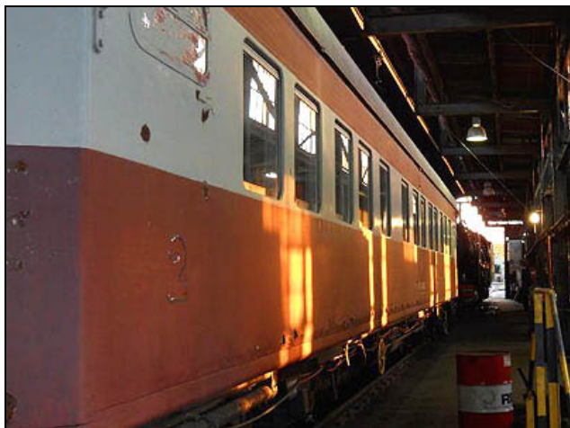
C07 – Now for the worse side! We are learning how to weld in patches on the rusted Sandstone Sleeper, using a combination of MIG, TIG and stick-welding for the job. So, the patchwork will not be so simple and straight forward.
