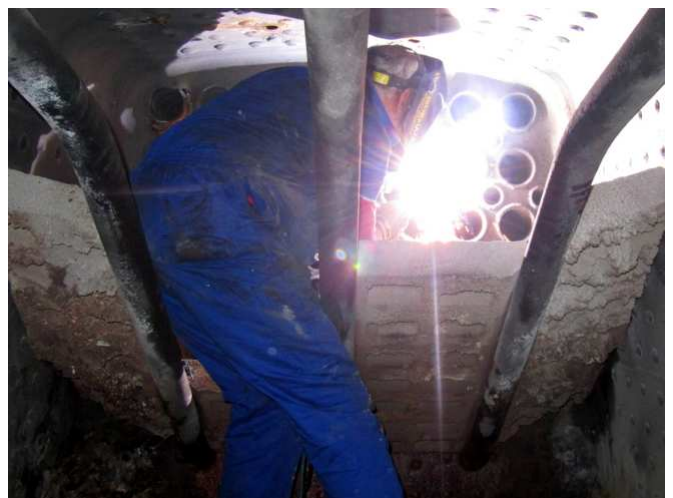
Boilermaker Alfie fixes some leaking tubes that keeps giving headaches. Right at the top is an empty hole for a fusible plug which was replaced by Brett and Michael. Photos: Luca Lategan
