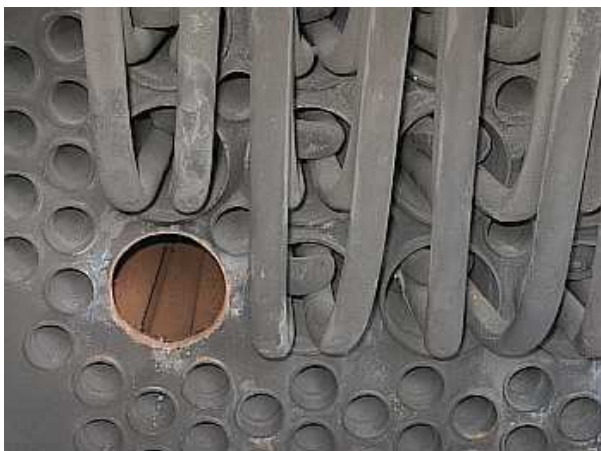
This shows where the faulty tube has been removed
