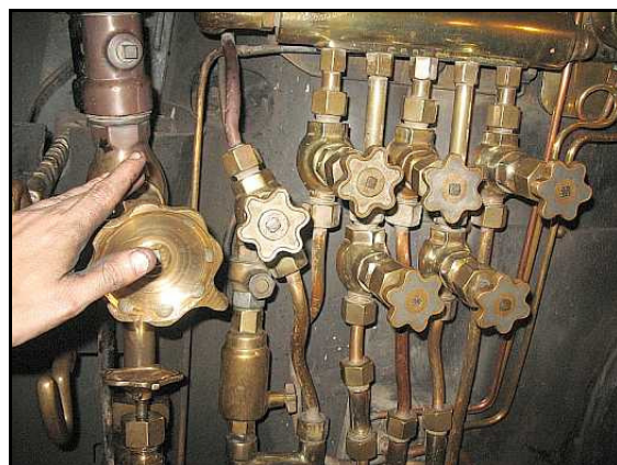
E07 – Quite a shopping list of salvaged brass valves and copper piping! These are the stoker jet valves, with the large valve to the left being the stoker booster, and the horizontal valve the stoker modulator valve.
