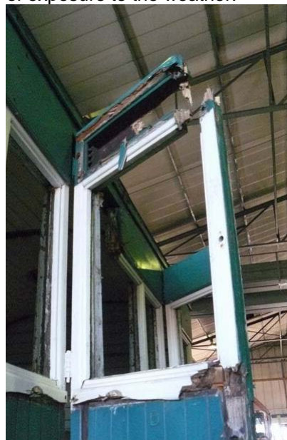
Wood rot on a door of coach no.83.
