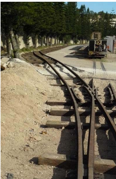
The lifted rails have been re-laid at the diesel depot. It is not known why this particular section has been laid on/next to the tared access road that leads to the rear of the diesel depot.
