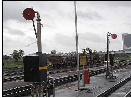
BS30 – In the foreground is a diesel refuelling station, with red disk targets showing the swivelling heads and the black enclosures protecting the flow meters. In the background is our mobile 'fuel depot', the DZ wagon full of coal and the hydraulic coal grab wagon.
