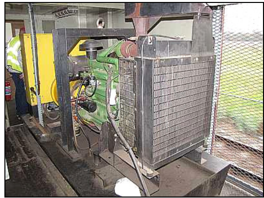
ST07 – The 85KVA generator set that had to be installed to handle the extra load of the electric geysers and enhanced lighting. The engine itself ran faultlessly, but we had problems with water contamination within the diesel fuel and the whole tank had to be drained and refilled on Saturday. But it's become a tradition to have generator and electrical troubles on a long trip – while the vintage, supposedly unreliable, steam locomotives just take everything in their stride.
