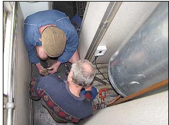
ST09 – The geysers fitted by the failed Setimela company are of low quality and were giving us trouble already on the outbound trip. Several of the circuit breakers were running close to thermal capacity and tripping out occasionally, aided and abetted by the long duty cycle required by ridiculously small heating elements in the large tanks.
