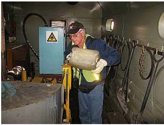
FP21 - Today's Safety Officer Tony "Shakey" King tries hard not to put extra bubbles in the water stream as he tops up the expansion tank of the diesel generator, prior to starting it up. (LG)
