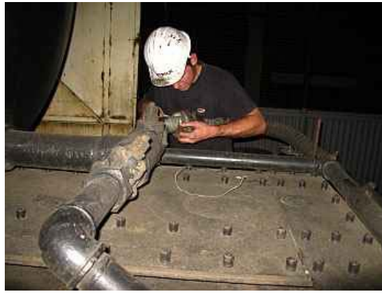
FP06 - Patrick wrestles with a slightly distorted bell coupling in our first attempt to make up a transfer water hose. Notice it's an old brake pipe that he's putting on. We were going to take three tankers and one hose turned out too short. We ended up with a stiff reinforced hose, a barrel and a converted brake pipe, which eventually had to be tied up with wire to keep it from sagging and swinging too much.
