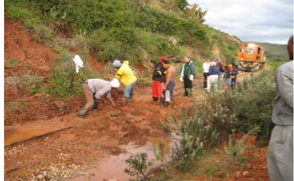
Clearing the mud slide.
